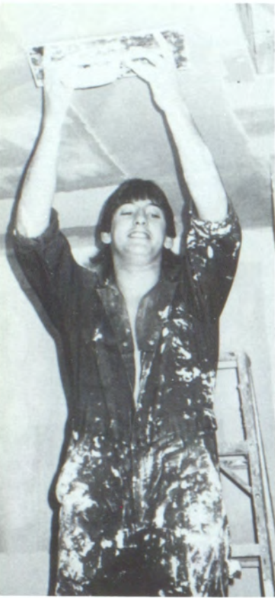
Josh Arthur puts spackling on the ceiling of the house they're constructing in Building Trades class. The house had a two car garage.
